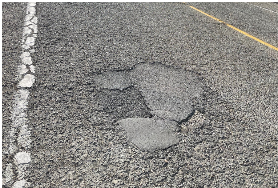
Photo 2: Section 2 Raveling, Alligator Cracks and Failed Patching
