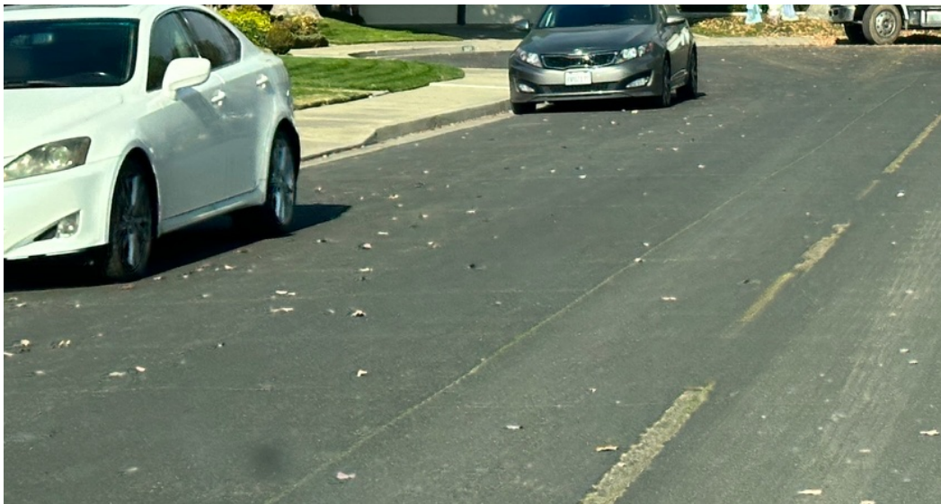
Photo 1: Section 1 Moderate Longitudinal Cracking
